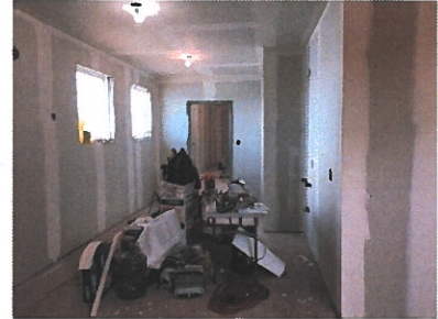
Drywall in process of mudding backstage. Dressing room A looking towards Dressing Room B (the Green Room). Windows look out to the harbour. Staff.
